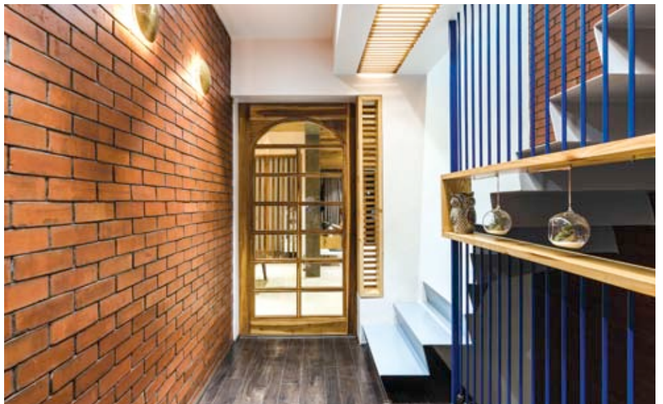
The shaft for the lift has been replaced with 5mm folded MS plate staircase.
